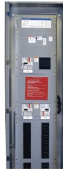
Wall-mount maintenance bypass panel
